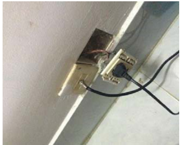
Damaged electrical sockets require immediate repair
