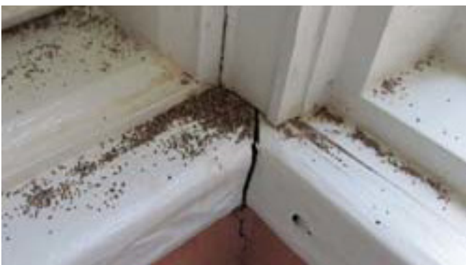
Mud deposits are a sign of active termites
